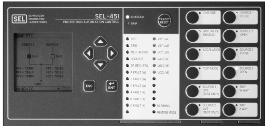
▲ ATC 451 control panel.
