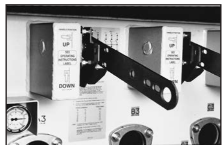
▲ Single phase interrupter operating handles.
