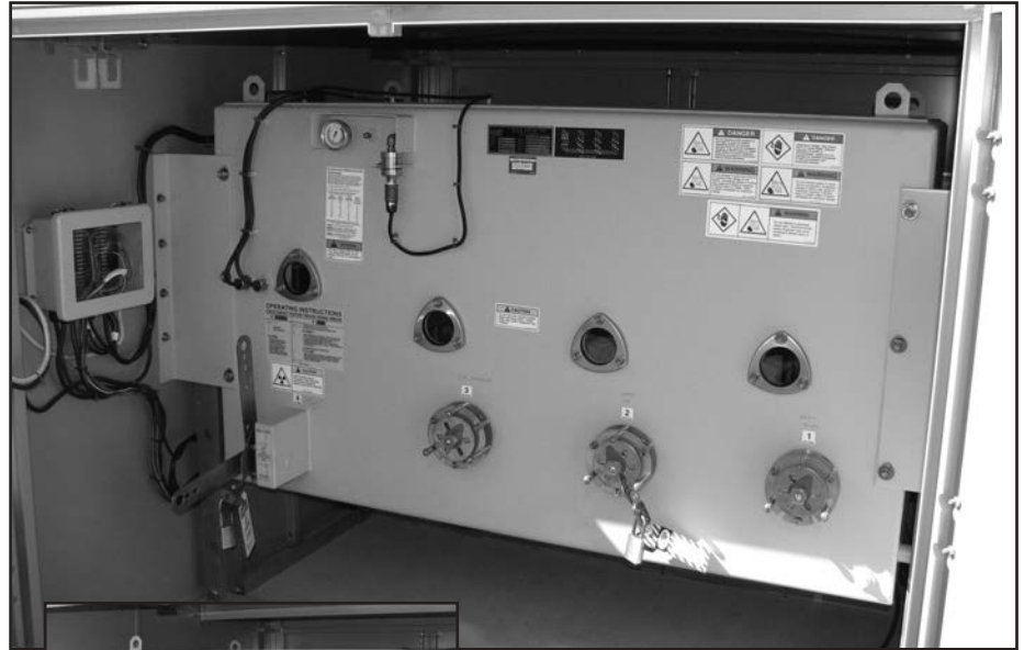
▲ Front and back view of a padmount PNI-43L with rotary style load break operator.
