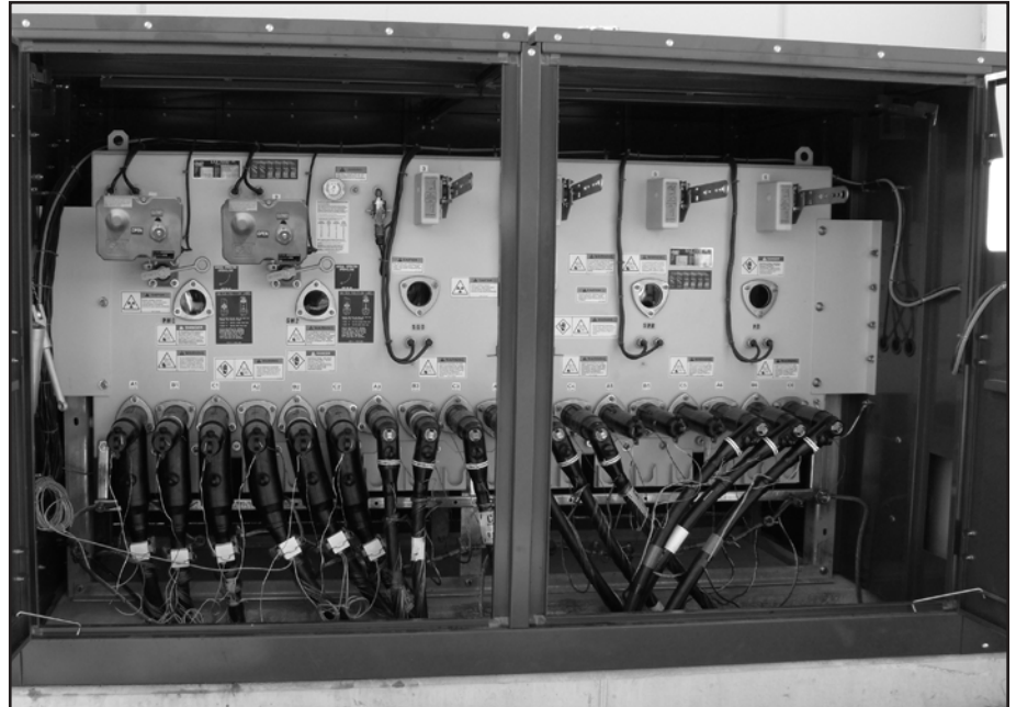
▲ Padmount switch with SEL controls.
