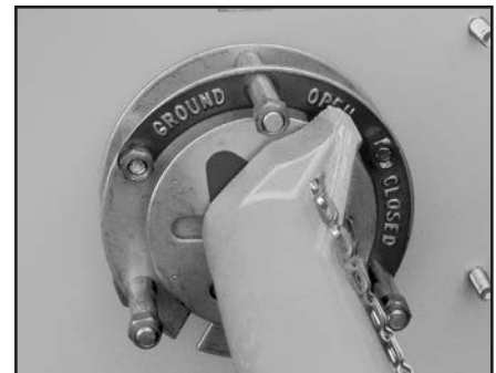
▲ Load break multi-position switch operator.
