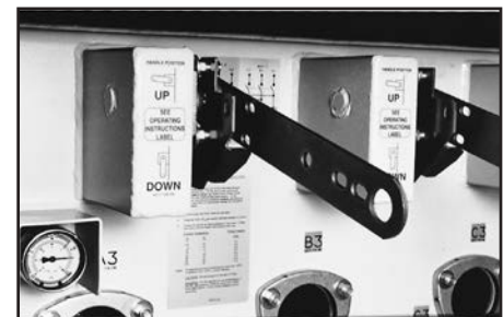
▲ Single phase interrupter operating handles.
